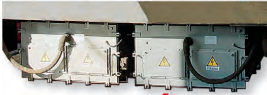
Power assemblies and converters for electric traction system
