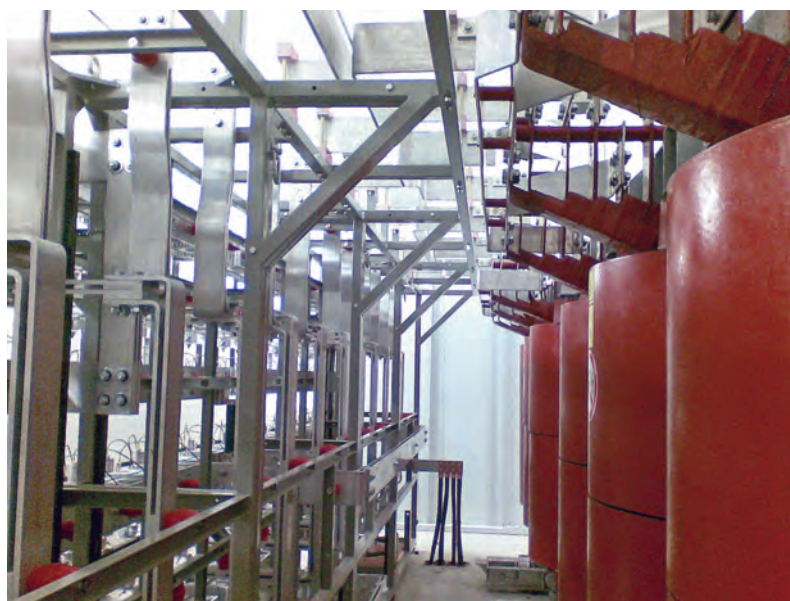
RAILWAY application 6.6MW 1500V 24 pulses Complete rectifier group: rectifier + transformers including bus bar connections among them
